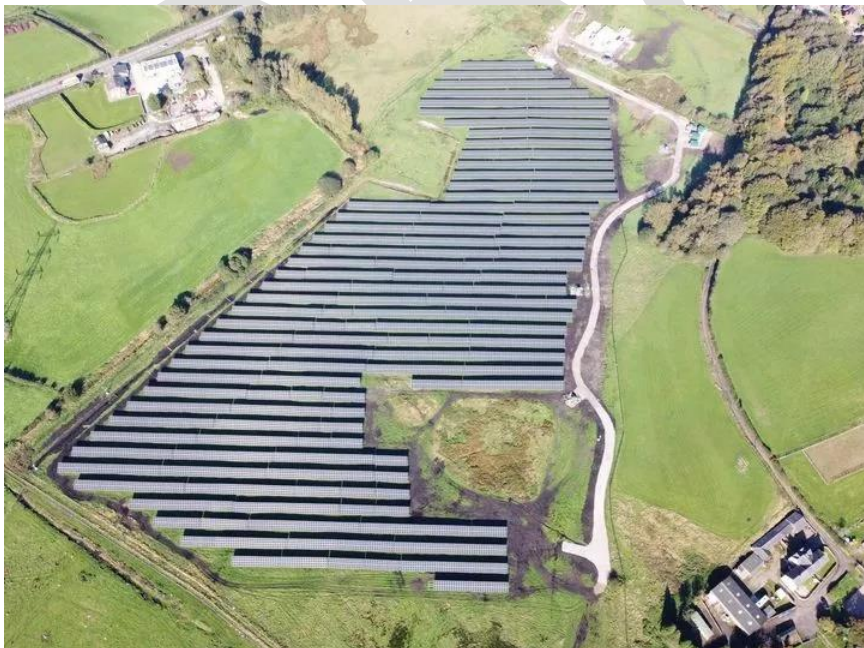
Fig. 7 Rochdale Council's 5.5MW Chamber House Solar Farm will provide enough electricity that could power 2,000 homes.
